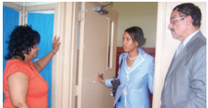
Councilmember Bowser reviews the needed repairs at MacFarland Middle School with Principal Antonia Peters and Council Chairman Vincent Gray.
